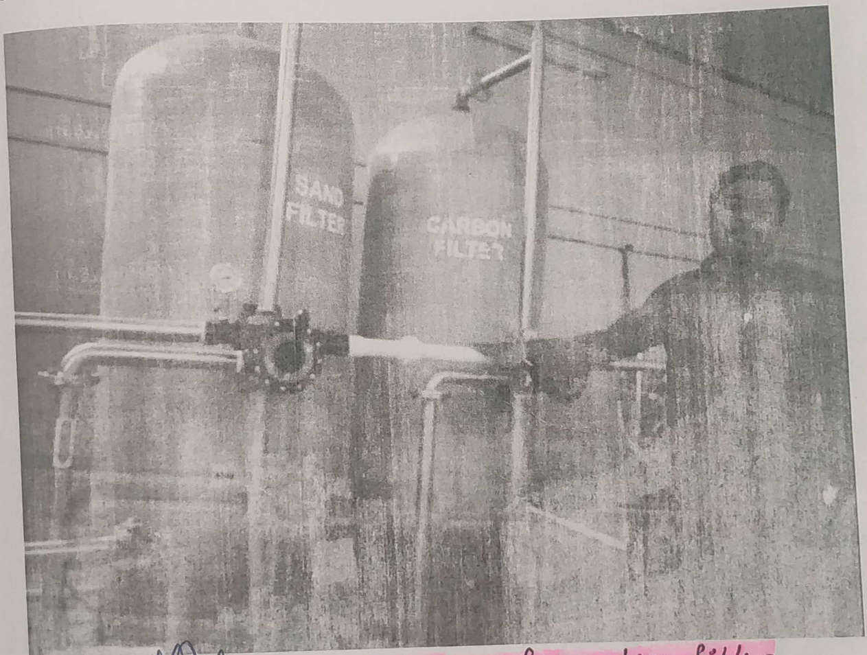
Picture of water filter
