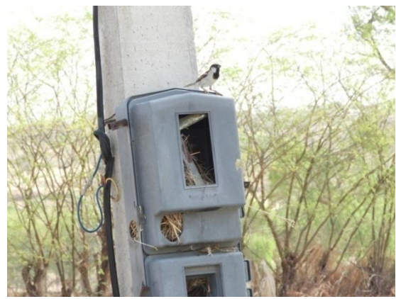
Figure 16: House sparrow nesting inside electric meter box
