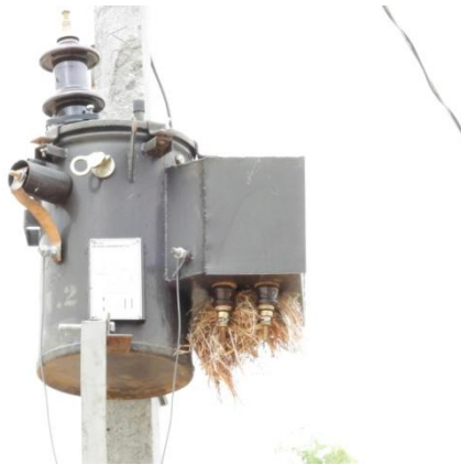
Figure 15: House sparrow nesting inside electric transformer
